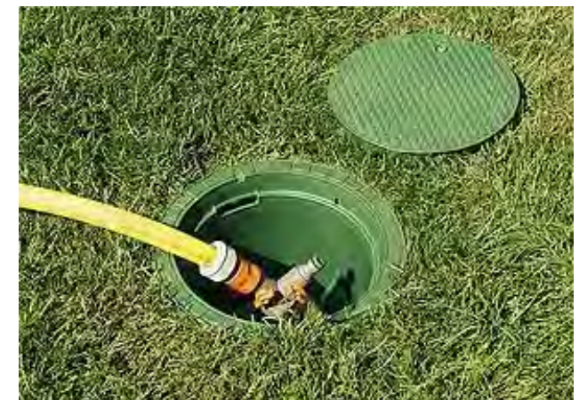
A ground-hose connection box
